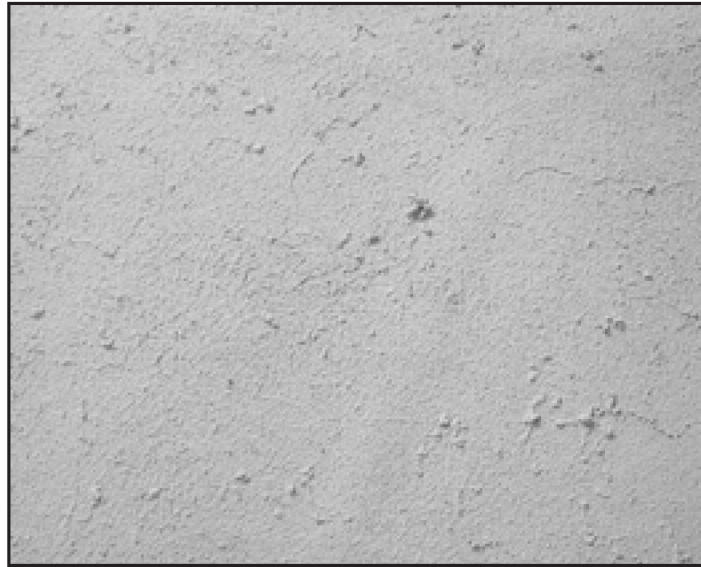
Photo 2. Example of over-mixing.
