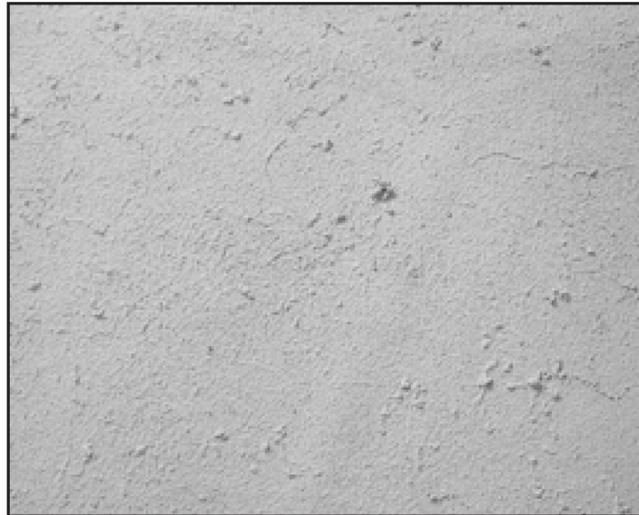
Photo 2. Example of over-mixing.
